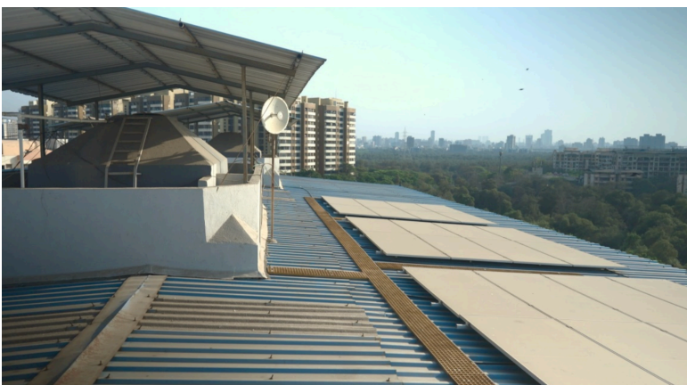
Figure 2: Rooftop solar panels installed at Nav Yuwan Housing Society
