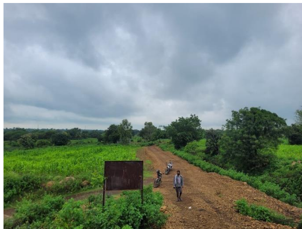
Figure 06: Silt from desilting of the pond repurposed to construct roads in Ainapur Village
