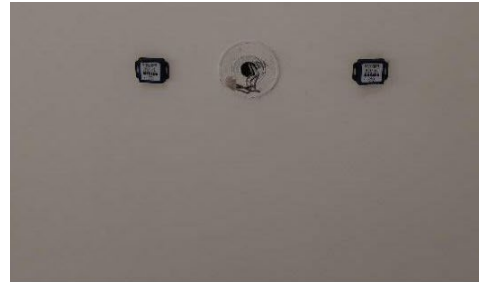
Temperature sensors installed for underdeck temperature measurement
