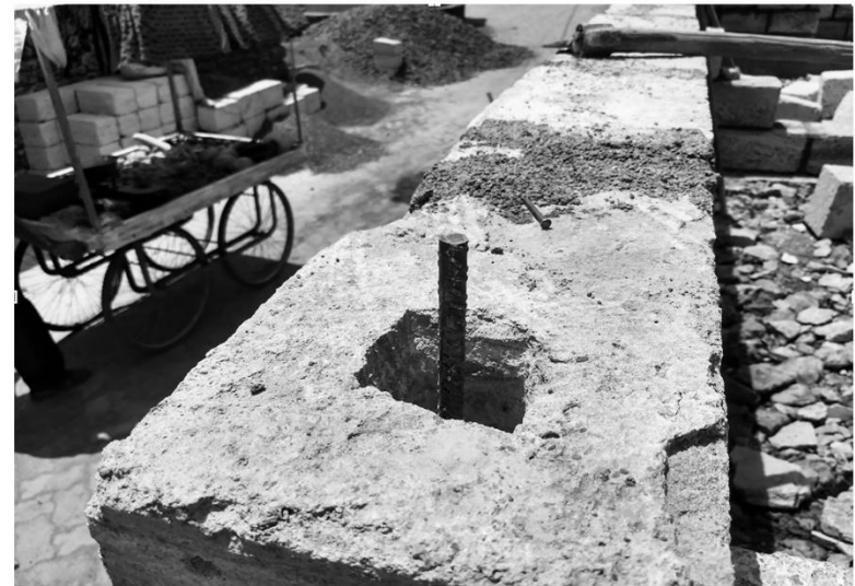
Fig 3.36 Optimizing the use of concrete - Ductile reinforcement inserted in cornerstones _Optimization feature 3
