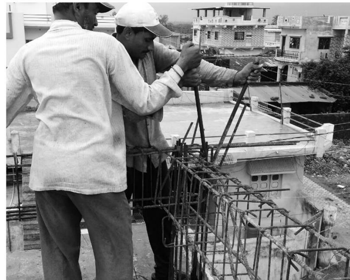
Fig 3.20 Mason training on Beam reinforcement bending, as a part of on-site practical session_Chitradvad (2017)
