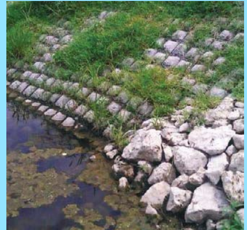
Figure 29 Image showing slope stabilization in French Broad river bank in Tennessee, USA
