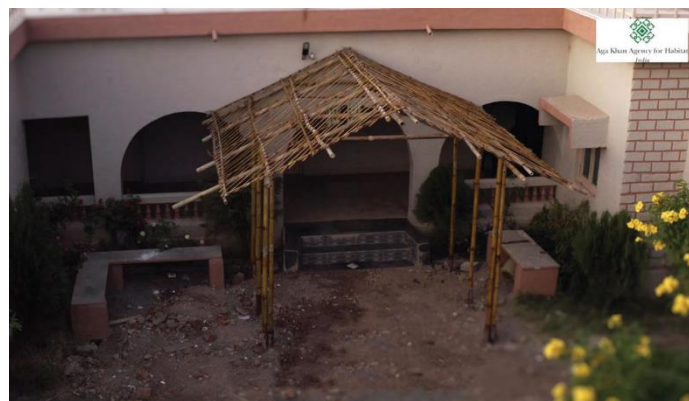
A demonstration of Bamboo porch constructed by AKAH field team with CGBMT's support at Habitat resource center Chitradav
