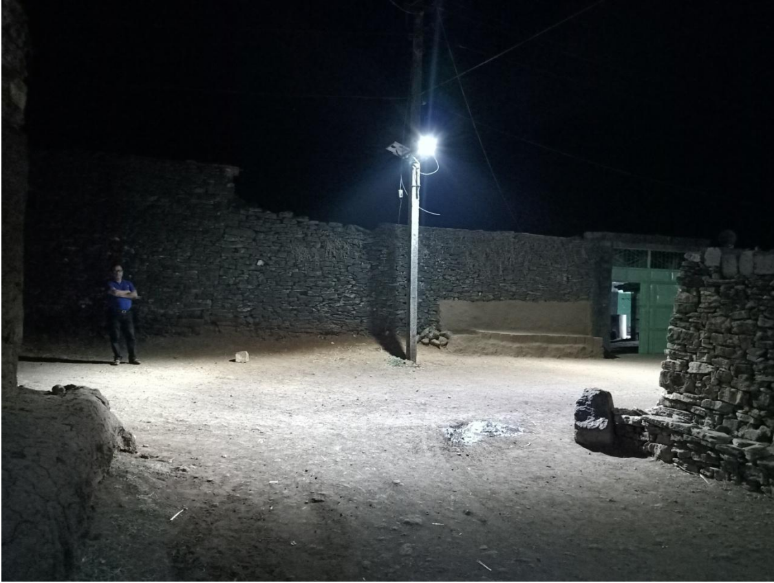
Solar light installed in one of the project villages by AKAHI
