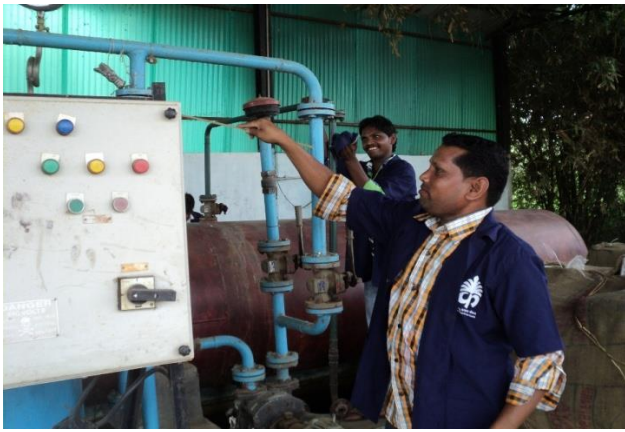
Bamboo Treatment Plant Operation
