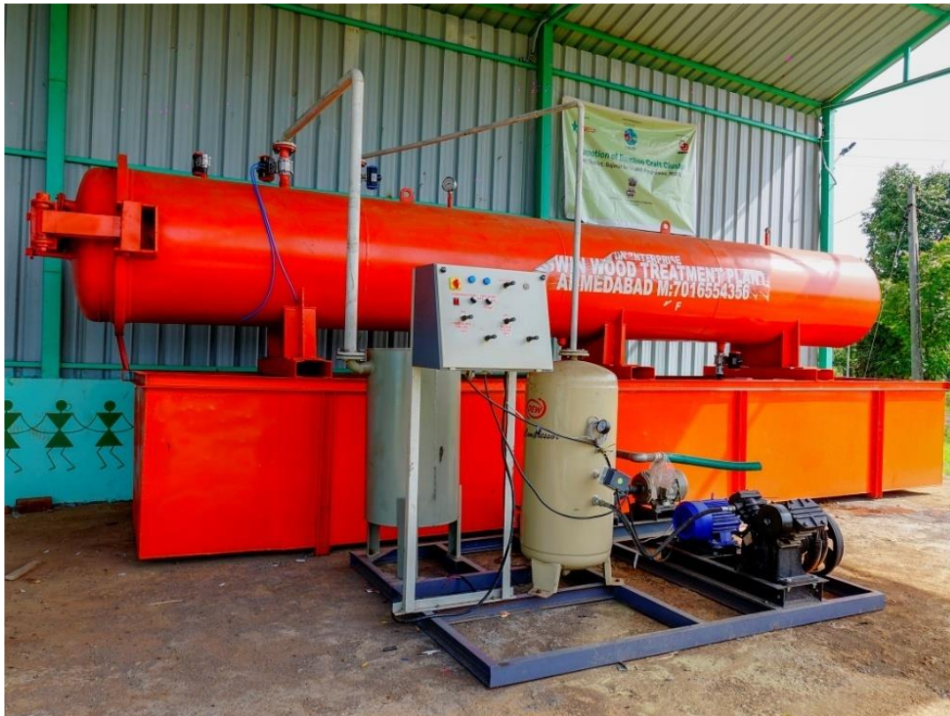
Pressure Vacuum Treatment Plant installed in CIBART facility
